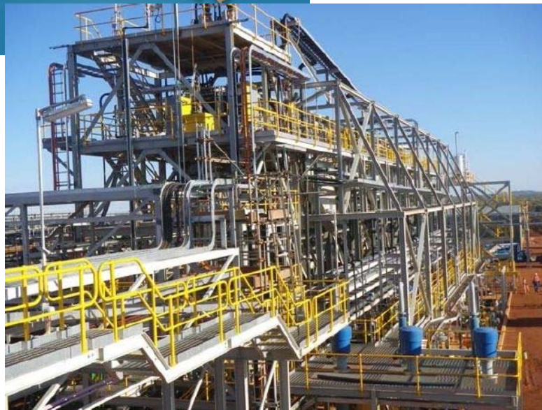
Mount Weld Rare Earths Concentration Plant
